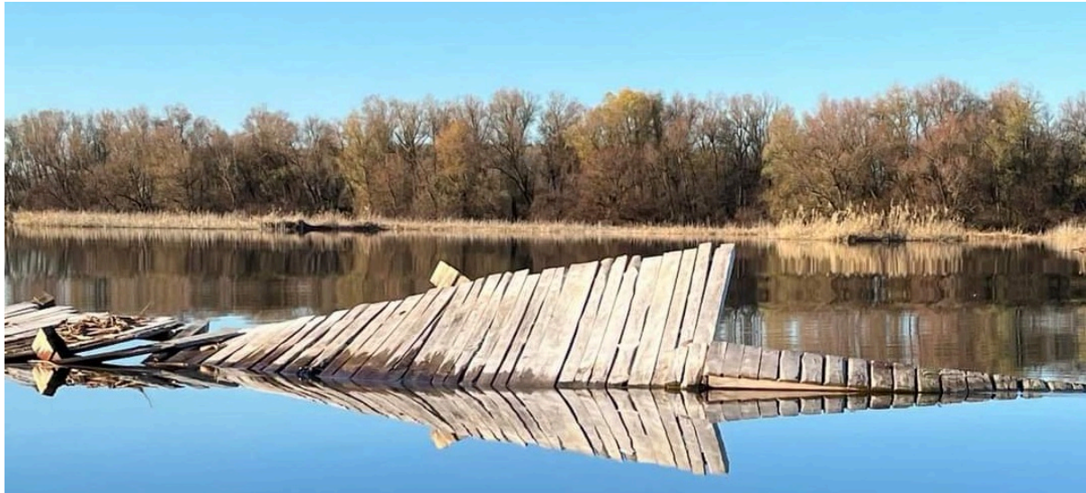
Figure 19. One of the destroyed platforms in Peschina Marsh, July 2023
